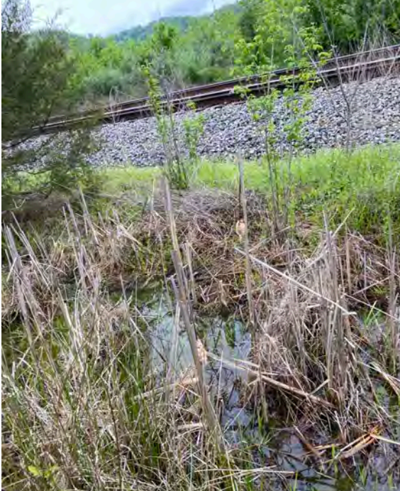
Photo 5- Water ponding found on the east side of the site near the railroad tracks
