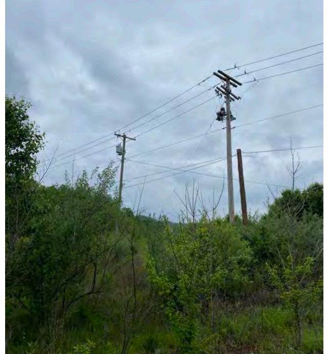
Photo 6- Pole-mounted transformers found on the target property
